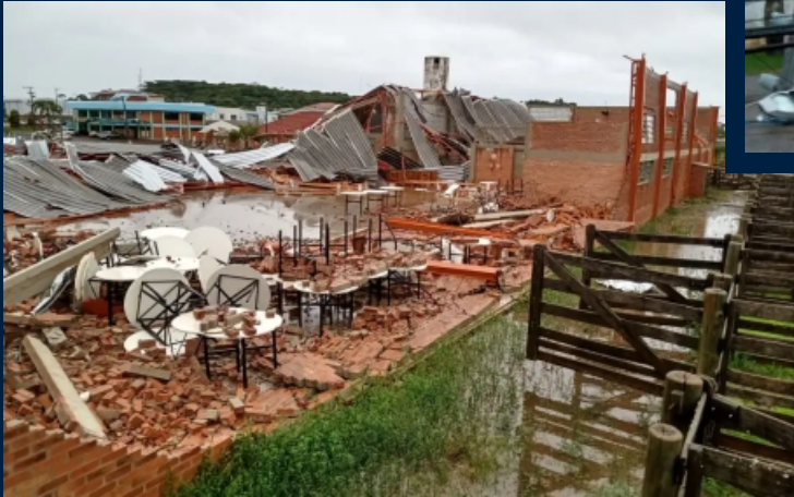
Warehouses in Muitos Capões, in the state of Rio Grande do Sul, destroyed by strong winds. Photo: Civil Defense of Rio Grande do Sul.
